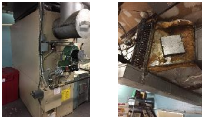
Figure 9- Furnace and Distribution
